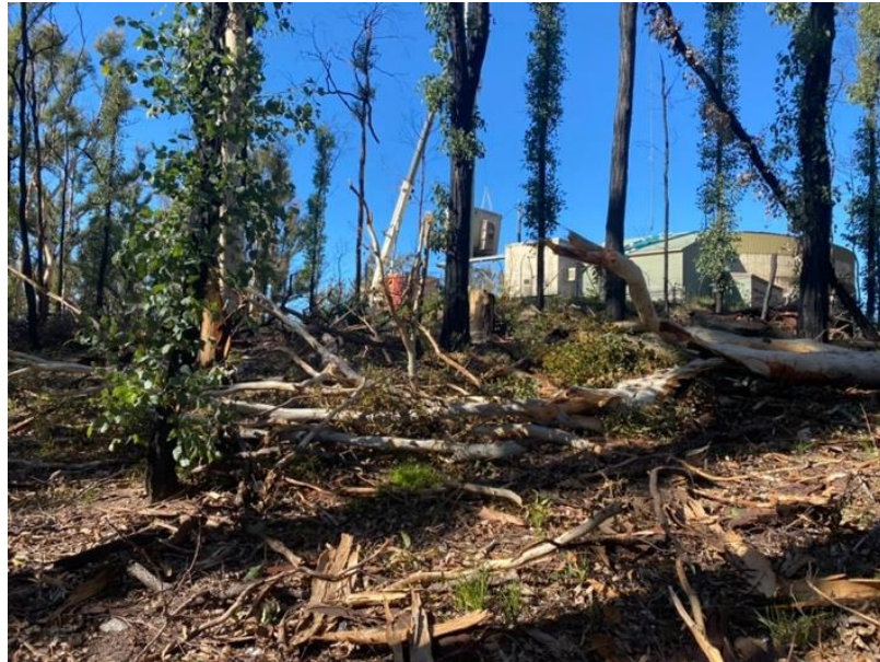
Figure 1: An under-construction APZ around the Malua Bay RFS shed. A crane can be seen in the background, replacing important communications assets destroyed by a fire on 31 December 2019. (Source Berkeley Braham, 2020)
