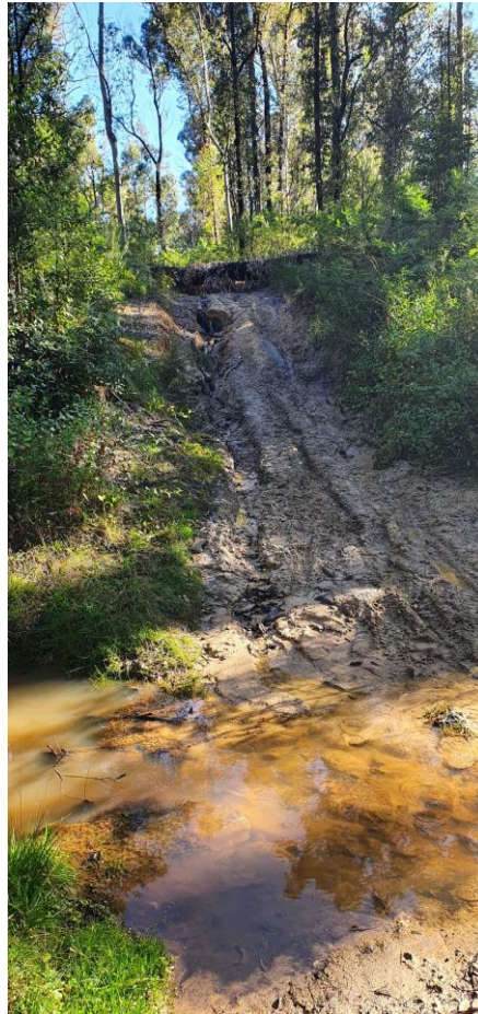
Figure 3: Washout and fallen tree blocking access on Cpt 150/2 in the Malua Bay RFS Brigade area (Source John Raymond, 2024).
